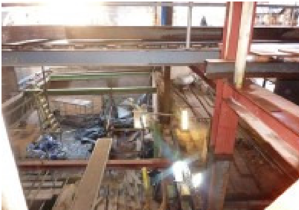
The work at height risks at the Mayfair site included missing edge protection to prevent falls.
